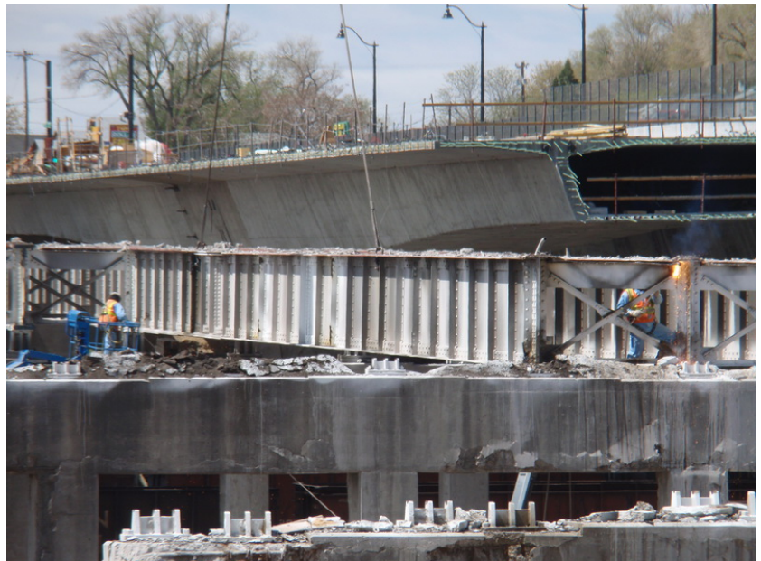
Figure 2 – Existing Bridge Demolition – May 7, 2010: A worker makes the final cut through a cross frame needed to remove a girder in Span 3 of the existing bridge. The girder is rigged to a 300-ton crane positioned on an access road in the rail yard. The main-span tip of Cantilever 3 EB can be seen on the right.
