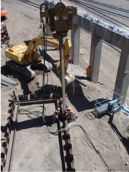
Figure 1 – EB Pier 5 Footing Excavation – May 5, 2010: A Flatiron crew drives sheet pile around the perimeter of the EB Pier 5 footing excavation area. The removal of girders from Spans 1 and 2 of the existing bridge was required prior to beginning foundation construction at EB Pier 5 and EB Abutment 6. An existing bridge pier is adjacent to the work area.
